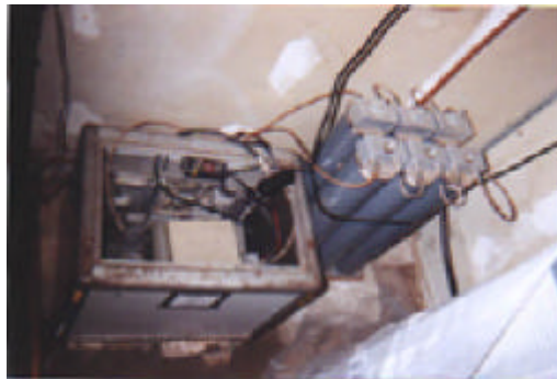
Overhead view of cramped quarters of repeater & duplexer
