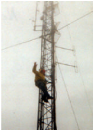
New repeater antenna at right
